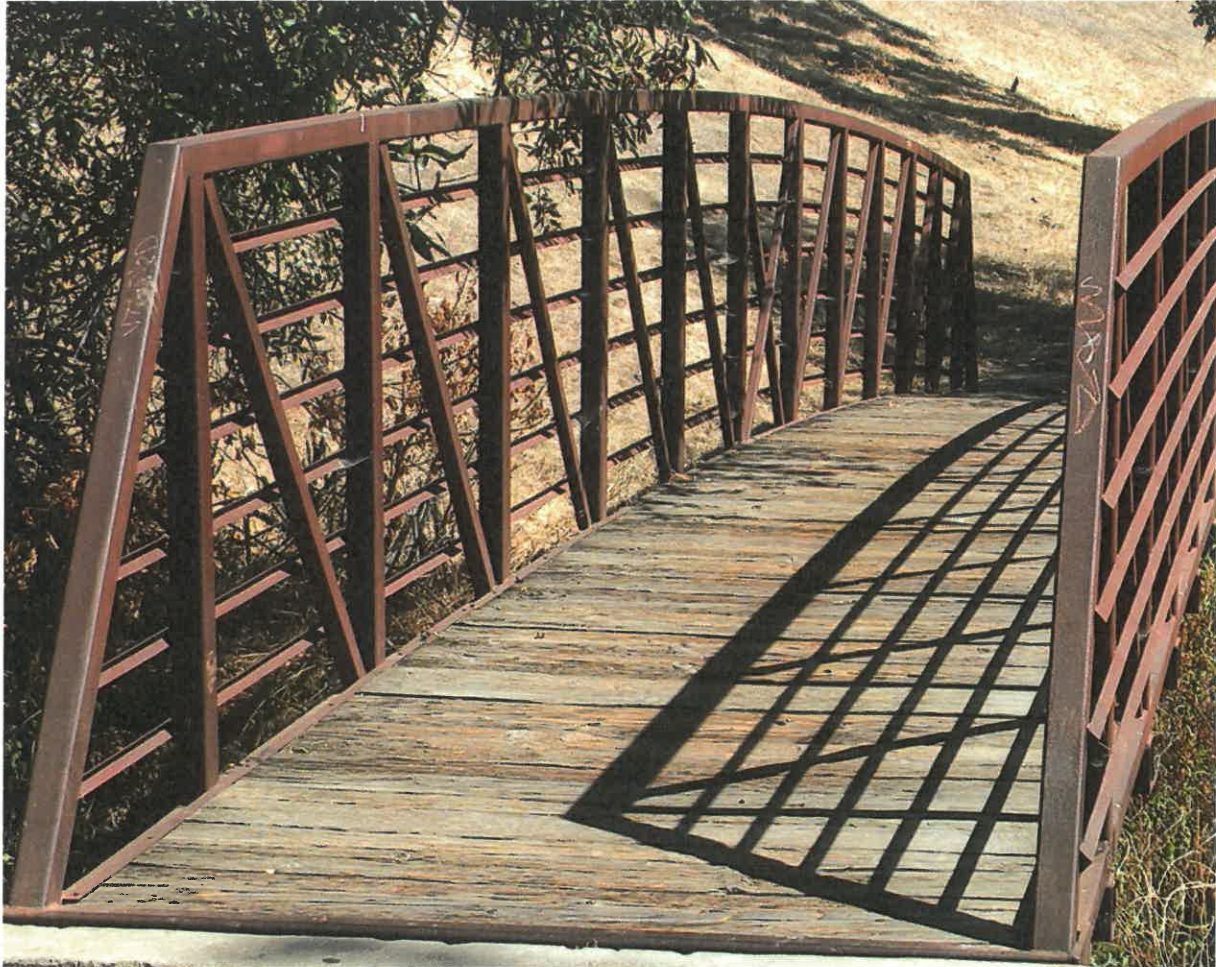
Before – decay wood
