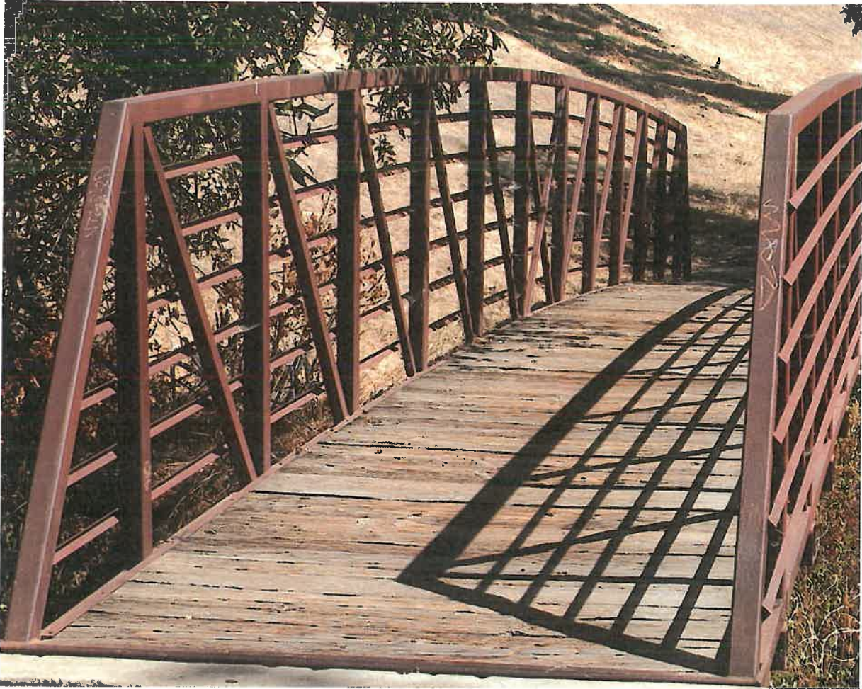
Before – decay wood
